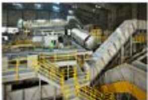
Material Recovery Facility - MRF
