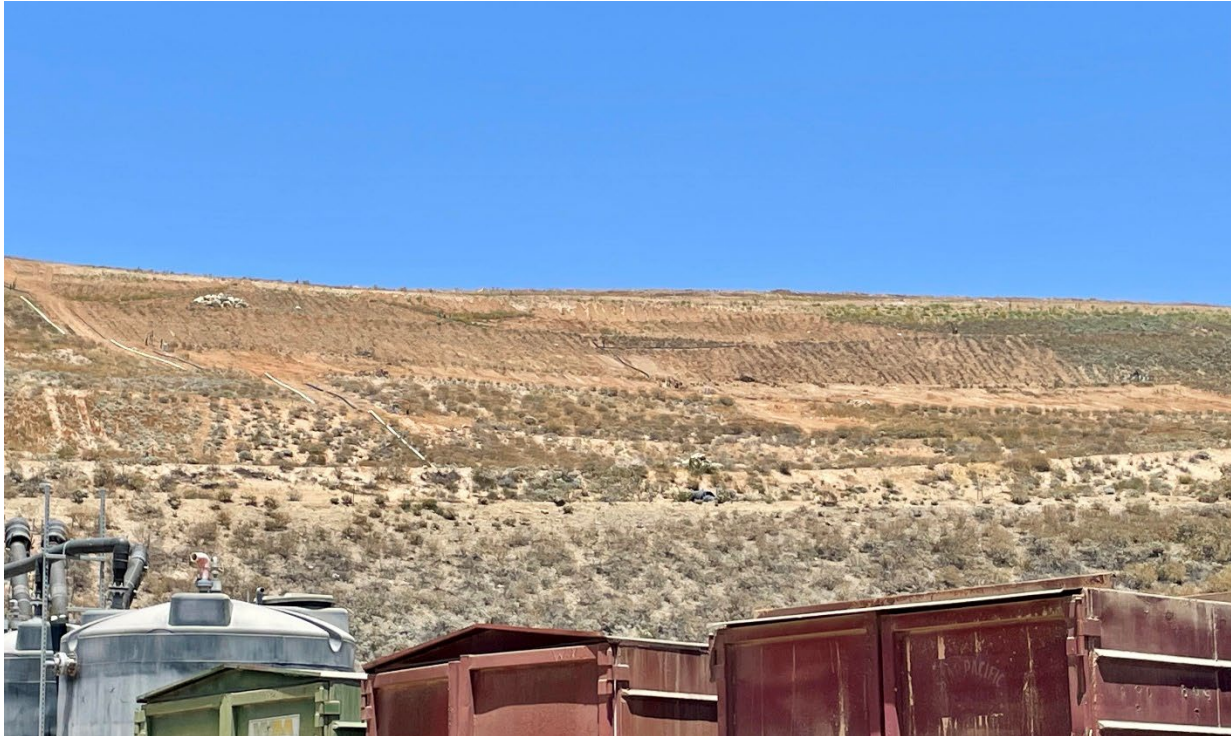
Photograph 20. Three slopes on Phases B2 and C1 were impacted for landfill repairs, June 22, 2023.
